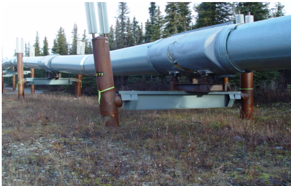
Figure 6 – Vertical Support Member (VSM) outward bending due to sideways impact
