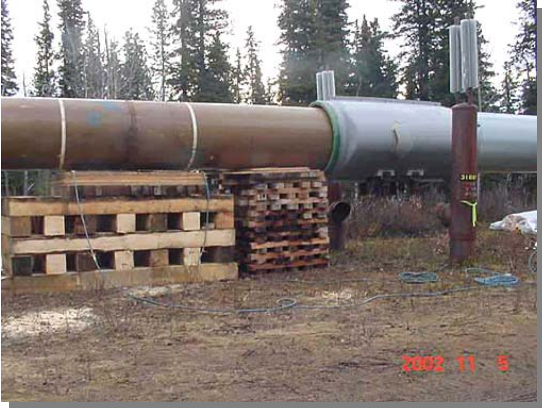
Figure 9 – Temporary cribbing under Trans Alaska Pipeline two days after event
