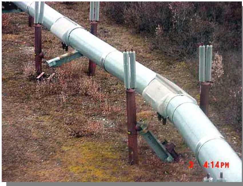
Figure 4 – Loss of two consecutive crossbeams due to near field seismicity just south of Denali Fault
