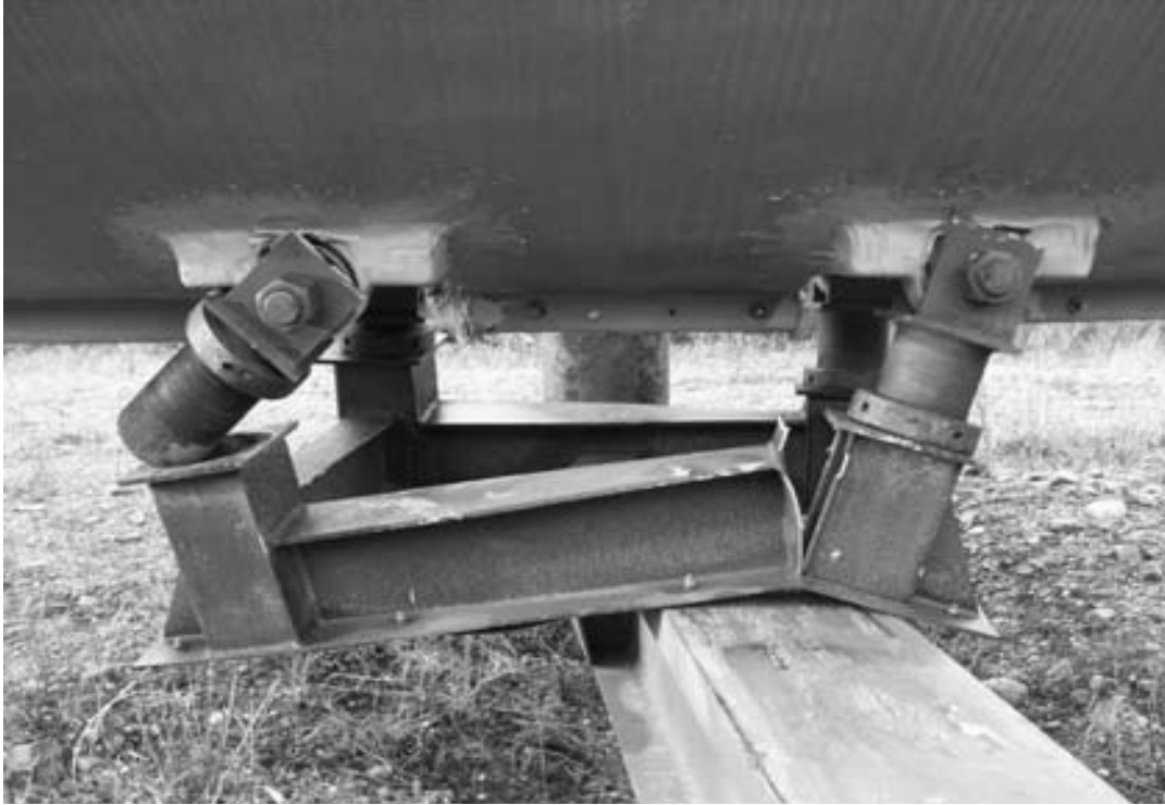
Figure 7 – Collapsed Shoe at VSM Bent
