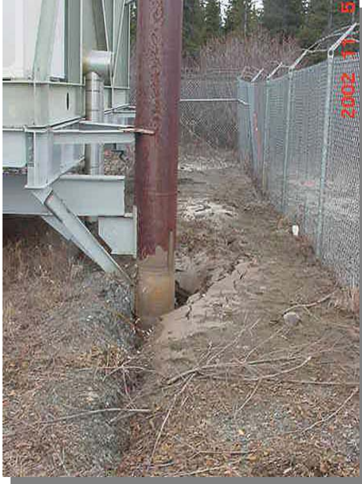
Figure 7 – Liquefaction at a Remote Gate Valve site (RGV 91)
