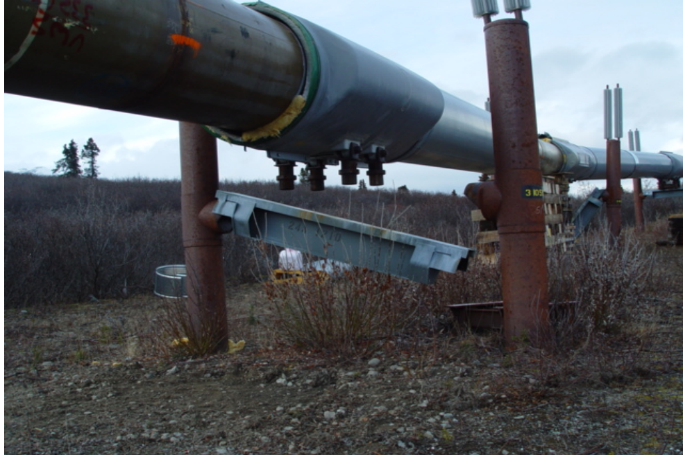
Figure 5 – Loss of Crossbeam and Shoe
